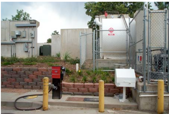
Figure 2. B20 Fueling Station
